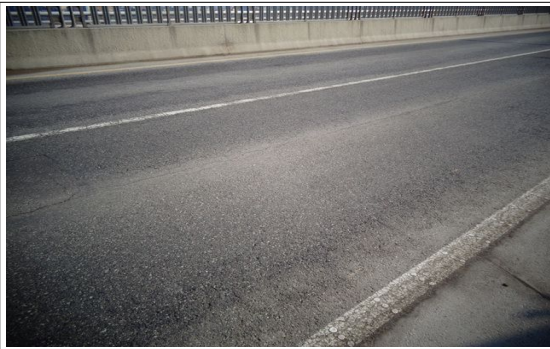
S11 망상균열 (원주방향)
